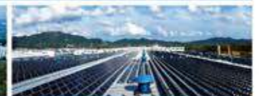
Solar panels arrays
